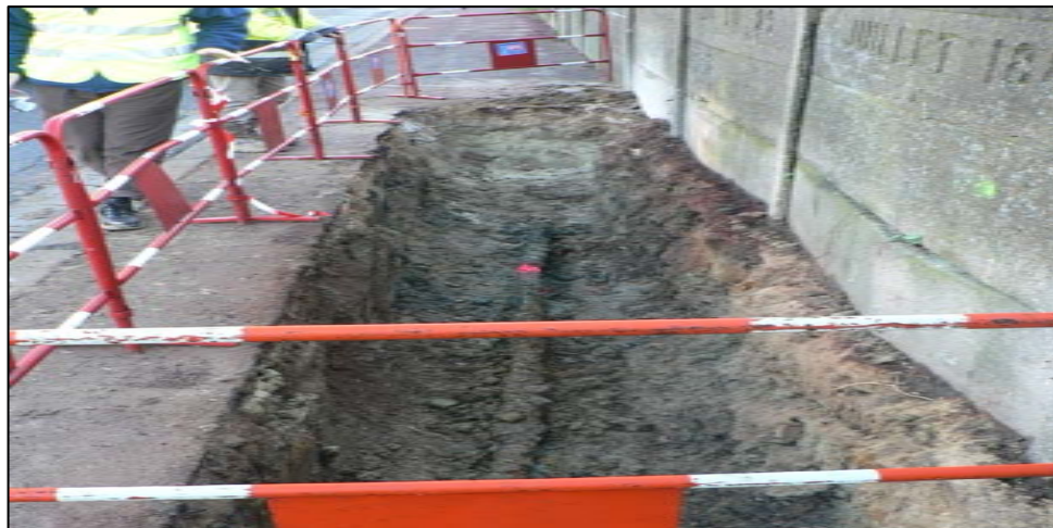
Soil excavation showing damaged cable
